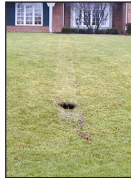
The sod is tamped back in place and all excess material is removed.
