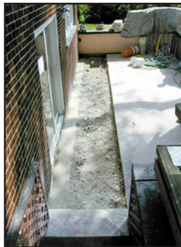
A grated trough drain solution was designed. The new drains are part of a system that carries water to the ditch in front of the house.
