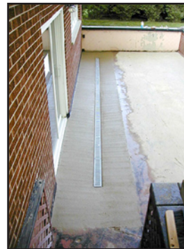
The finished drains have completely and permanently solved the problem. We use a heavier duty drain when installed in front of the threshold of a garage door.
