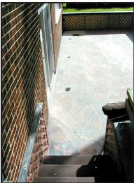
Existing drains could not keep up with heavy rains and customer's family room would flood.
